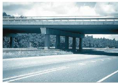
An example of a statically indeterminate beam used to support a bridge deck.
