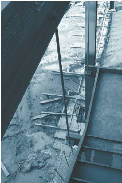
This steel tie rod is used as a hanger to suspend a portion of a staircase, and as a result it is subjected to tensile stress.
