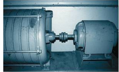
Stress concentrations can arise at the coupling of these shafts, and this must be taken into account when the shaft is designed.
