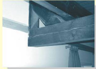
Typical shear failure of this wooden beam occurred at the support and through the approximate center of its cross section.
