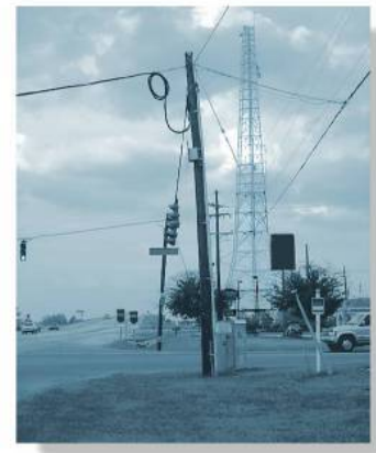
The long-term application of the cable loading on this pole has caused the pole to deform due to creep.
