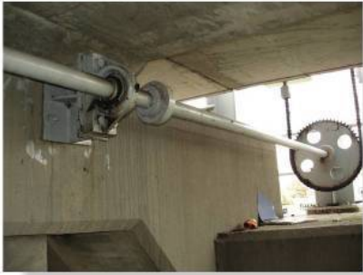
Long shafts subjected to torsion can, in some cases, have a noticeable elastic twist.
