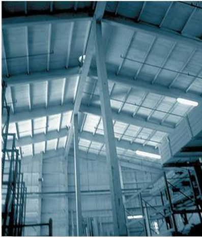
These long unbraced timber columns are used to support the roof of this building.
