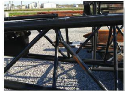
Failure of this crane boom was caused by the localized buckling of one of its tubular struts.
