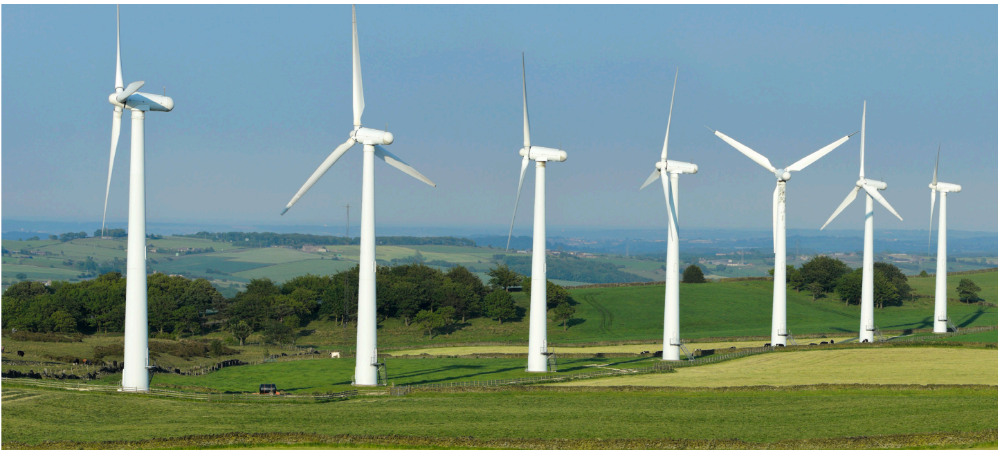
16-1. Typical wind farm.
