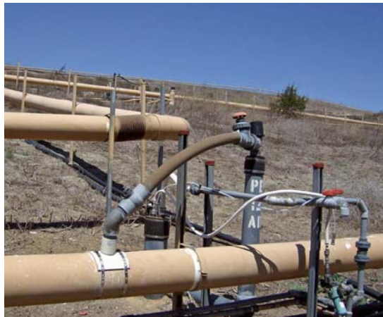
Methane well and gas collection pipes
