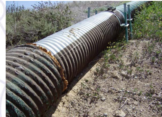
Storm water drain pipes
