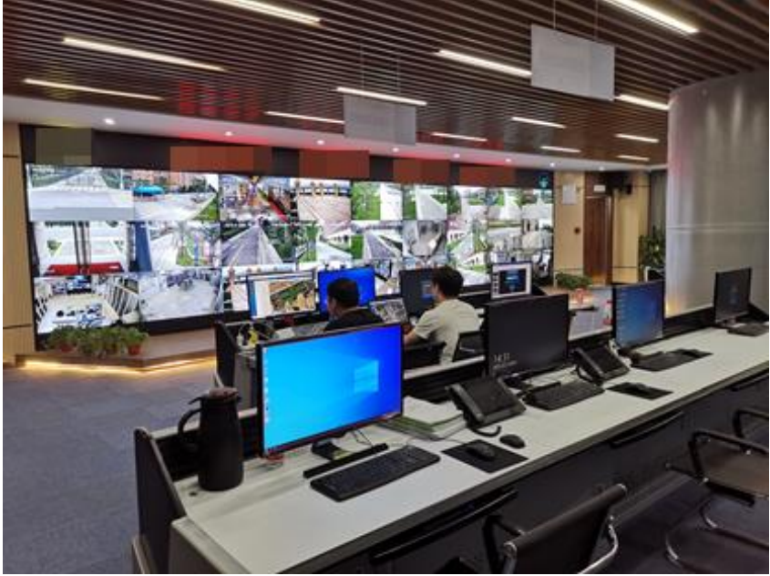
Figure 4-2 Example of the dashboard at the information control center
